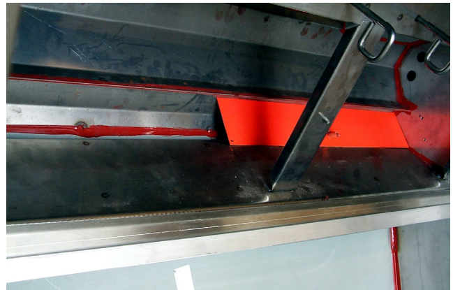
Fig. 3: First blank-off plate in a 2-fryer hood shown in final position. A second plate, needed to complete the installation, will overlap the first in the center of the hood.
